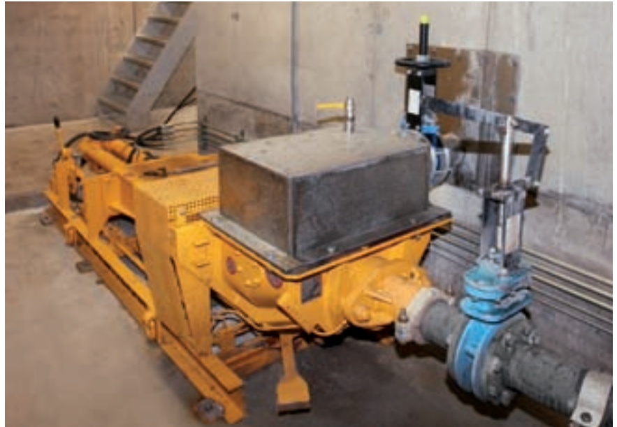
KOS 740 in biogas plant in Schlitters/Austria
